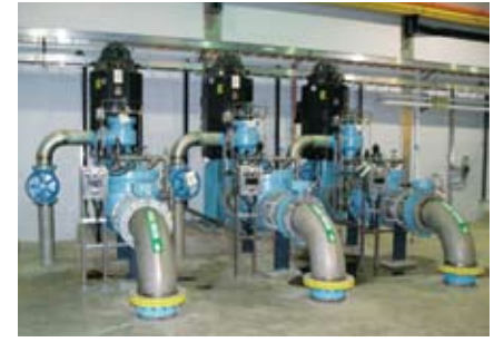
New Verticle Turbine High Lift pumps
