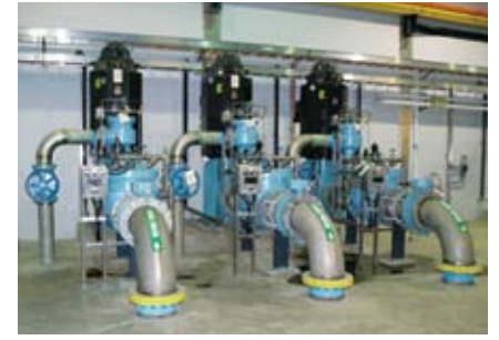
New Verticle Turbine High Lift pumps
