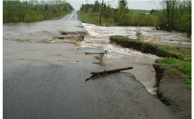
Example of storm damage (Highway 595)
