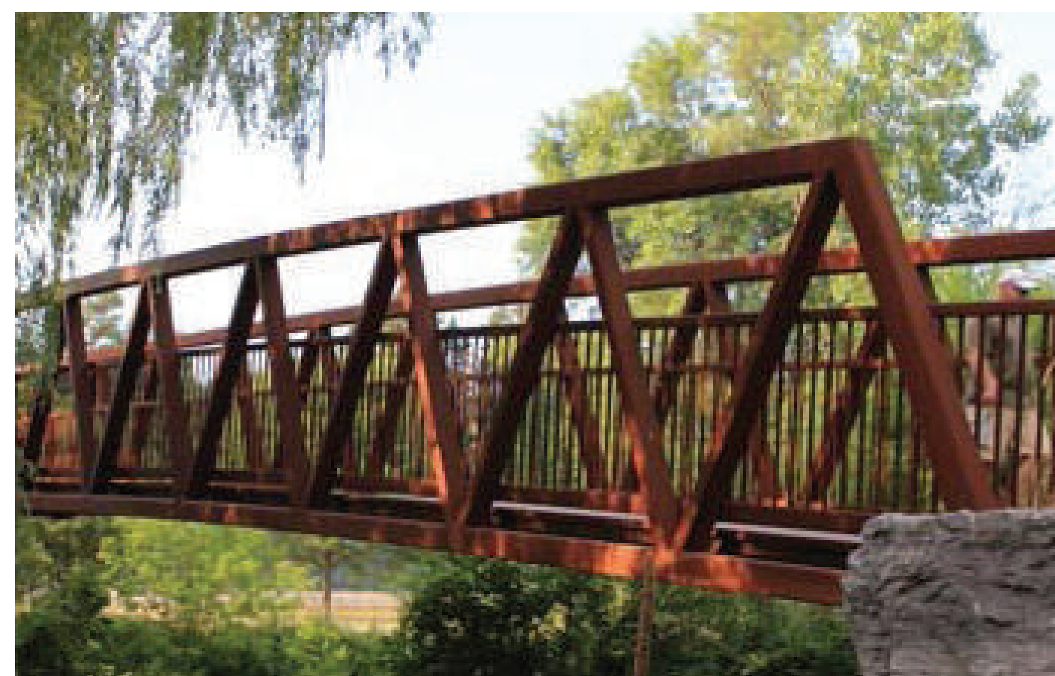
EXAMPLE OF WEATHERED STEEL WARREN TRUSS
